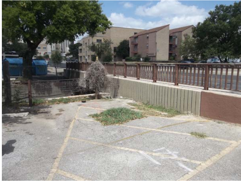
TRAVIS STREET (GATE UPSTREAM)
